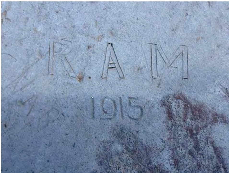
Figure 5: The initials of Rowland Arthur Marriott inscribed in the lead roof of Boynton Hall. 13
